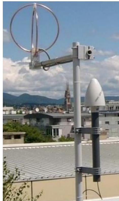
Fig. 3. LINET sensor antennas (orthogonal rings) and GPS antenna [14]
